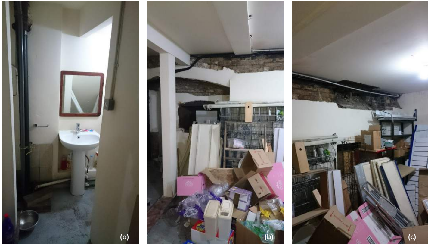
Figure 21 (a) - (c). Views of the basement storeroom. (a) View of the bathroom in the under-stair area with toilet (not pictured) situated around the corner.
