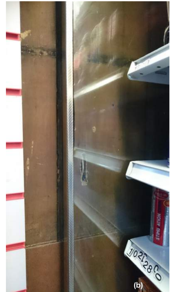
Figures 17 (a) and (b). Views of the wall finish behind the slatwall shelving system. See also Figure 18(b).
