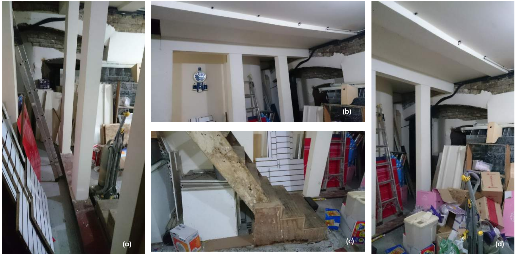
Figure 20 (a)-(d) Views of the basement storeroom with subsequent soffit and series of pillars resting on steel beam introduced to replace temporary props. Staircase introduced for access via the trap door.
