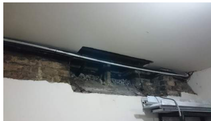
Figure 12. View of recessed area in western wall and ceiling, likely housed pavement lights in line with previous recessed entrance to shop.
