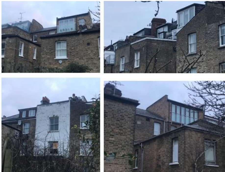
IEWS OF ROOF EXTENSIONS, FIRST-FLOOR EXTENSIONS AND ROOF BALCONIES FROM REAR GARDEN OF APPEAL SITE
