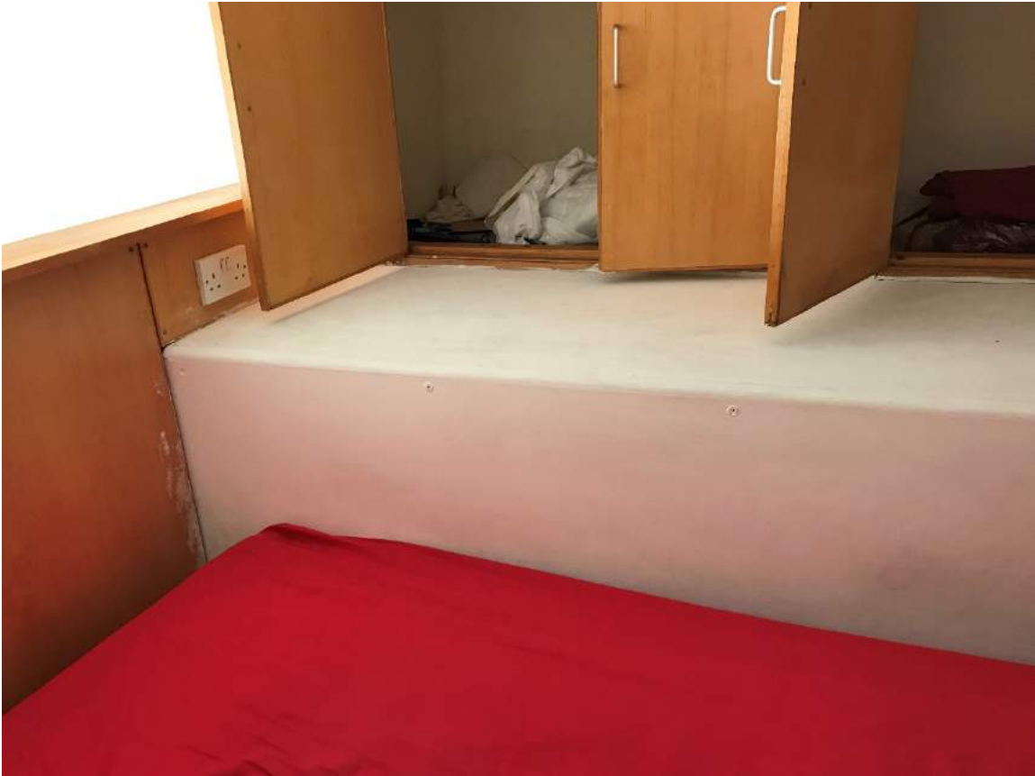
Figure 2: Services boxing on mezzanine levels to be removed as part of Phase 1
