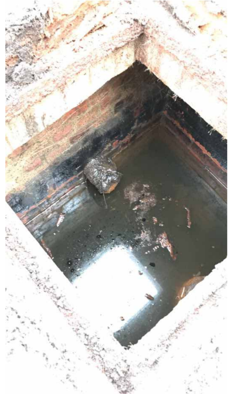
Three stage interceptor in south west Site corner
