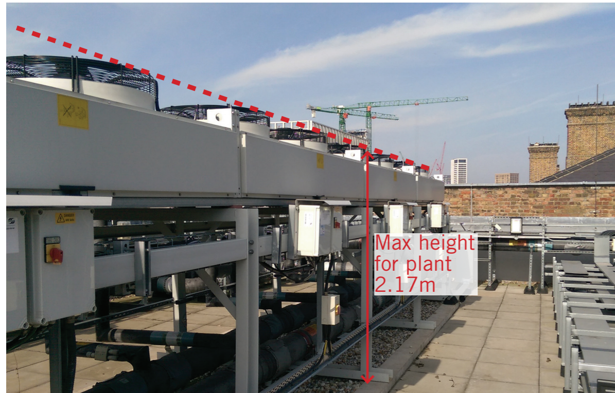
Fig. F.4 Central Block plant deck showing the maximum height of new plant
