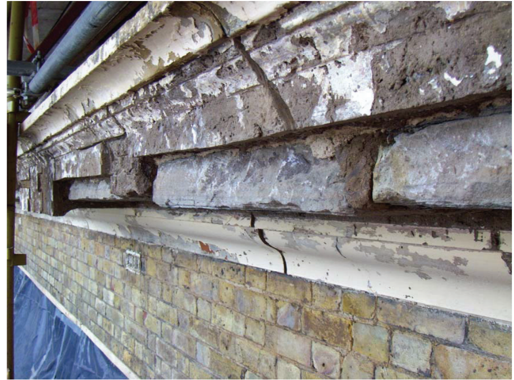
Photograph 2: showing the variation in the level of the stone soffit and the profile of the render moulding.
