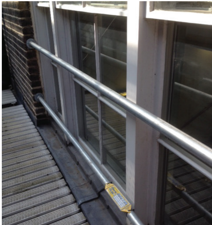
Fig. F.6 Example of safety railing across a window on the Western Range
