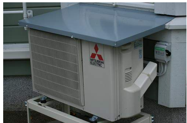
Figure 11: Outdoor unit of an ASHP
