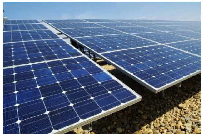
Figure 9: Monocrystalline PV arrays
