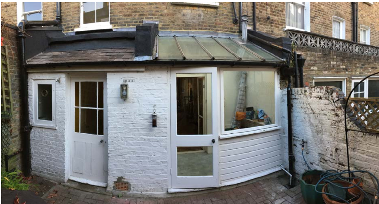
Existing brick extension on left of house, glazed extension to be replaced on right side. Description of Proposal
