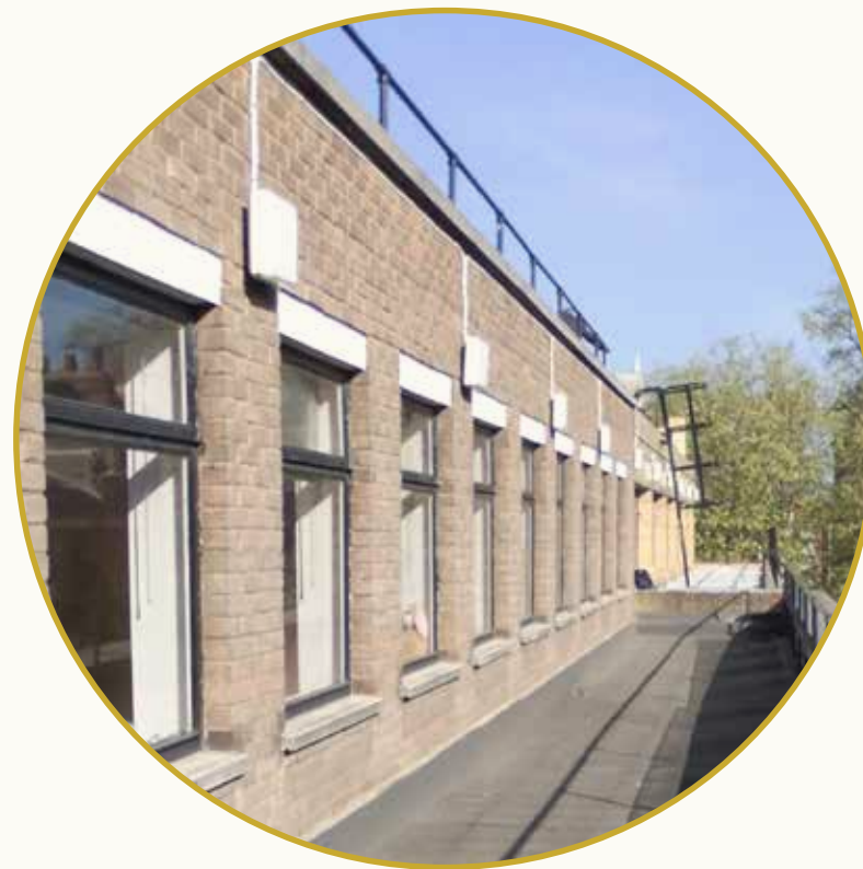
EXISTING LIGHT FITTINGS TO DANE STREET TERRACE.
