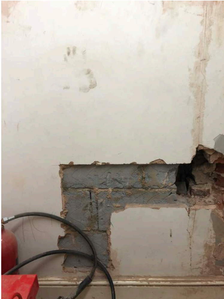
Fig. 4 Trial opening from No 15 showing former opening at 2 nd floor blocked with concrete blocks
