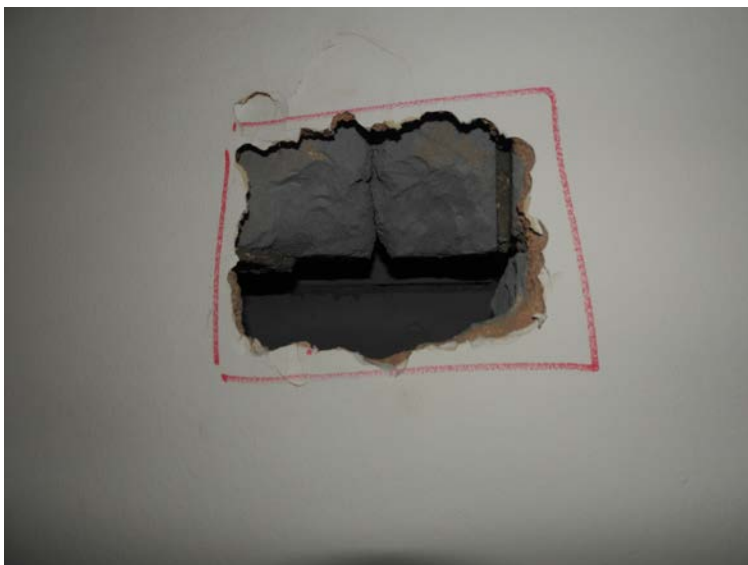
Fig. 5 Close up from No 14 showing concrete blocks infill of existing opening at 2 nd floor level
