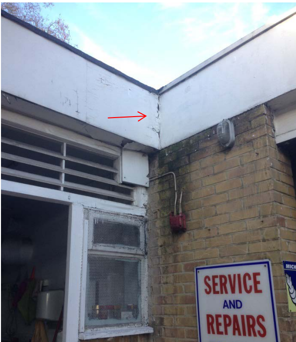
Photo 3: Small cracks in the corner of the soffit boarding.
