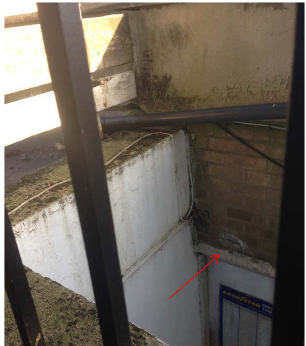
Photo 4: Superficial gaps in the brickwork on the northern aspect of the building.
