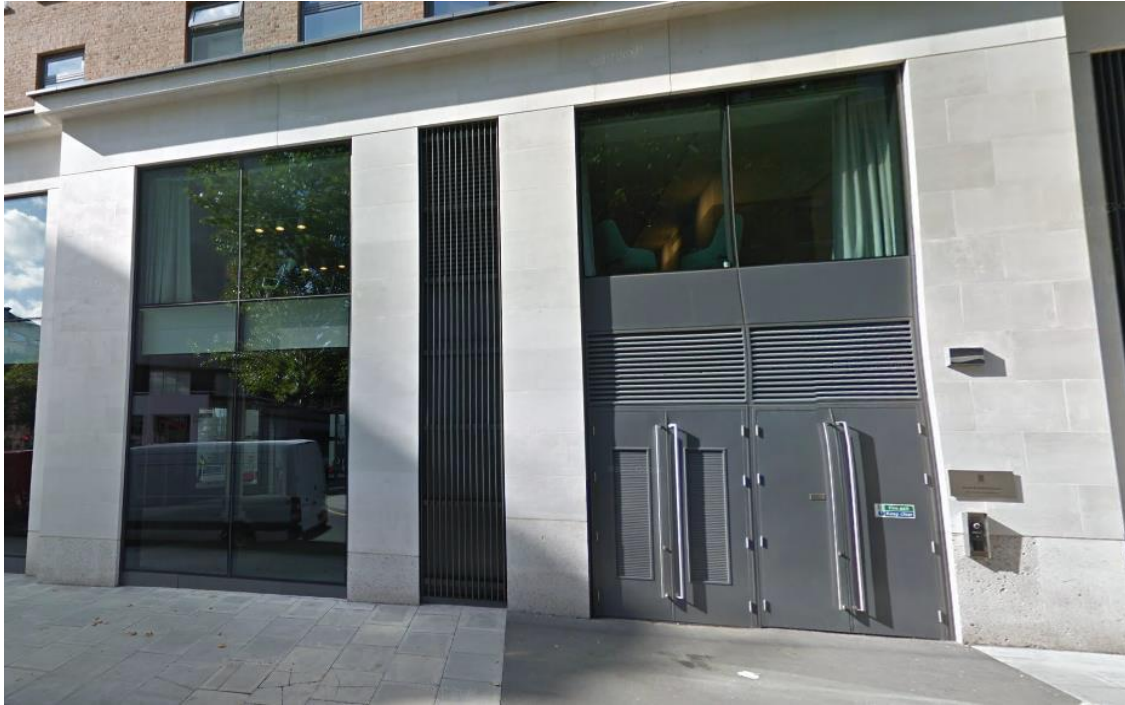
Photo of the East Elevation Louvres located on the ground floor (Bury Place)
