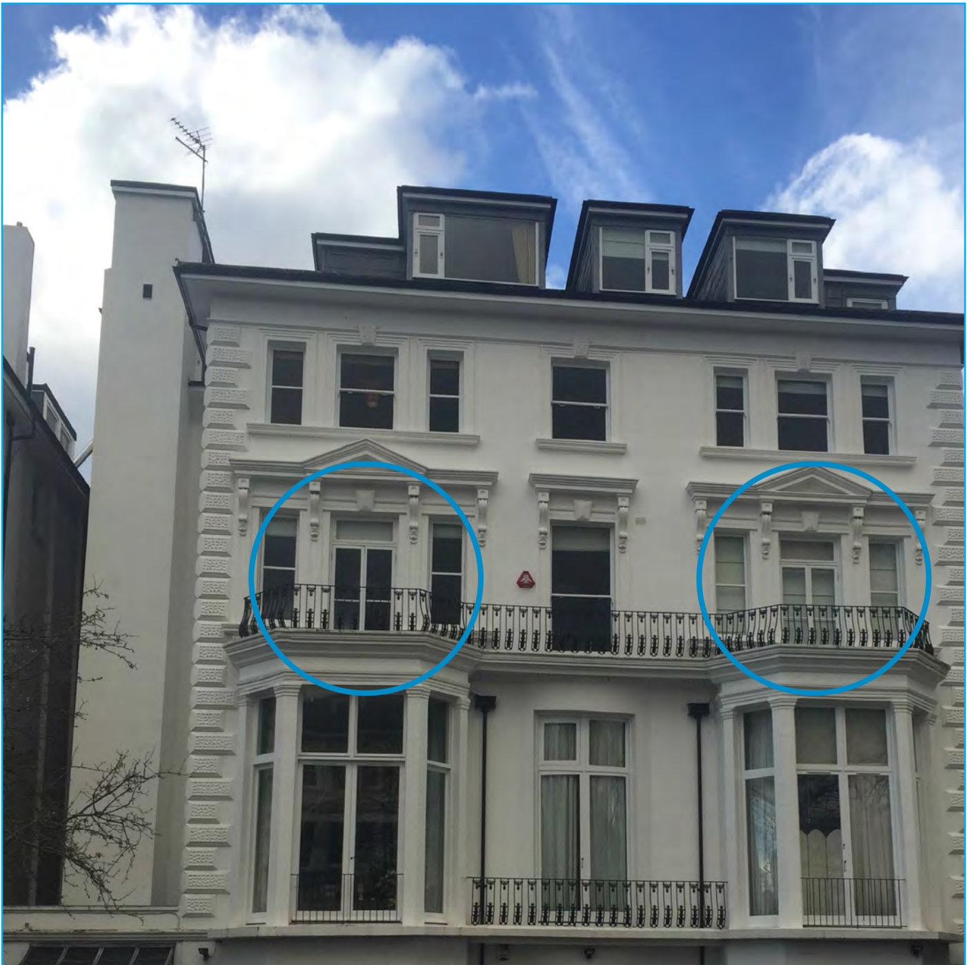
Examples of existing french doors and fixed panel above (matching our proposal) found in close proximity of the site: No. 3 Belsize Grove. Here the balcony is also extended.
