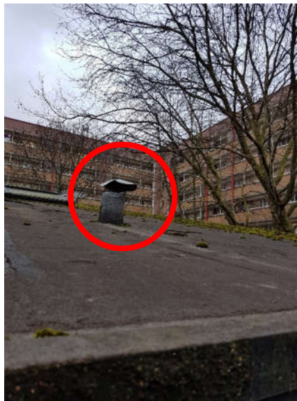
Figure 4-1 Atmosphere-side fume extract duct termination above the roof of the existing workshop at Old Tenants Hall.
