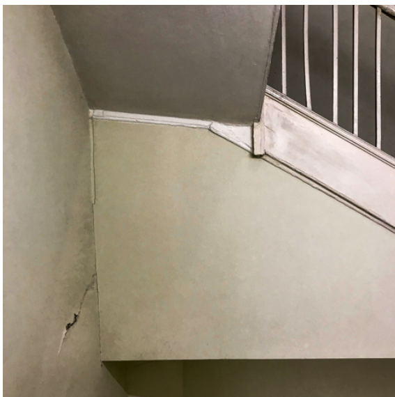
Image 6, View of Small Staircase Damage
