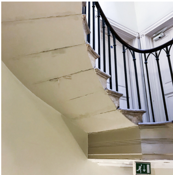
Image 5, View Internal Staircase Damage
