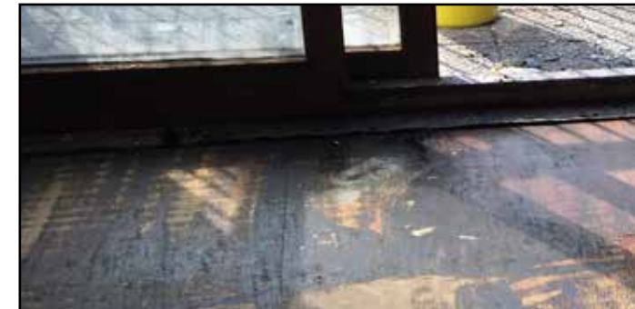
Photo below: ingress of water to floors below Example of constant damp through to flooring under carpeting
