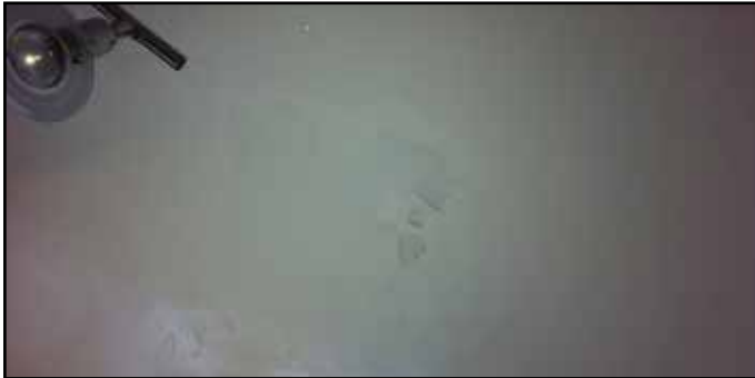
Photo below: ingress of water to floors below Example of constant leaking through ceiling below
