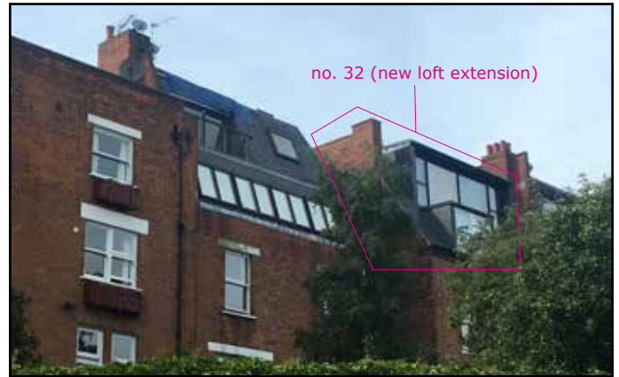
Photo below: showing existing balcony door, July 2017 No.30 needing repairs and no.32 built extension with aluminium frames
