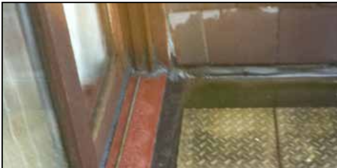
Photo below: constant external repairs insufficient to keep out infiltration
