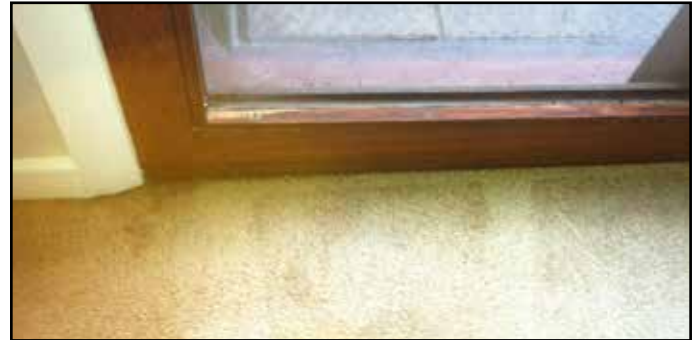
Photo below: water infiltration and degeneration of frame Example of constant damp on timber, carpeting
