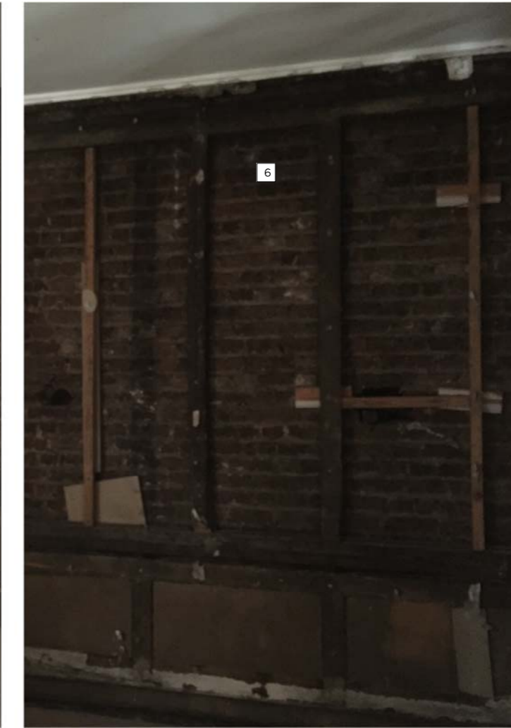
700_601 08 Example of existing timber panelling needing full refurbishment Master En-suite r1.03
