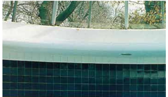
17. Existing Perimeter light trough
