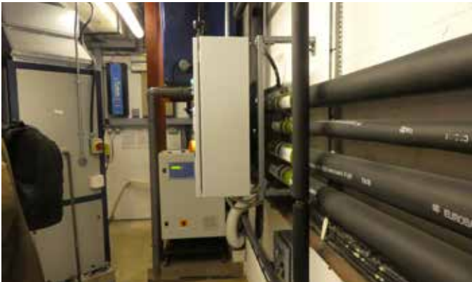
15. Existing Pool Plant
