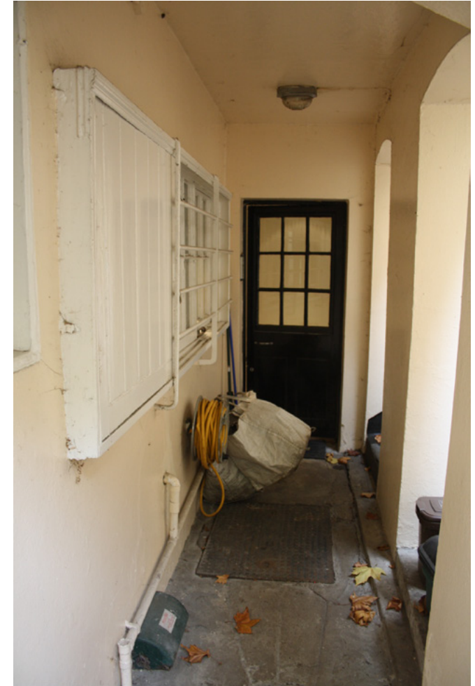
Covered area with arched openings in north elevation, with the basement kitchen window visible to the left of the photograph
