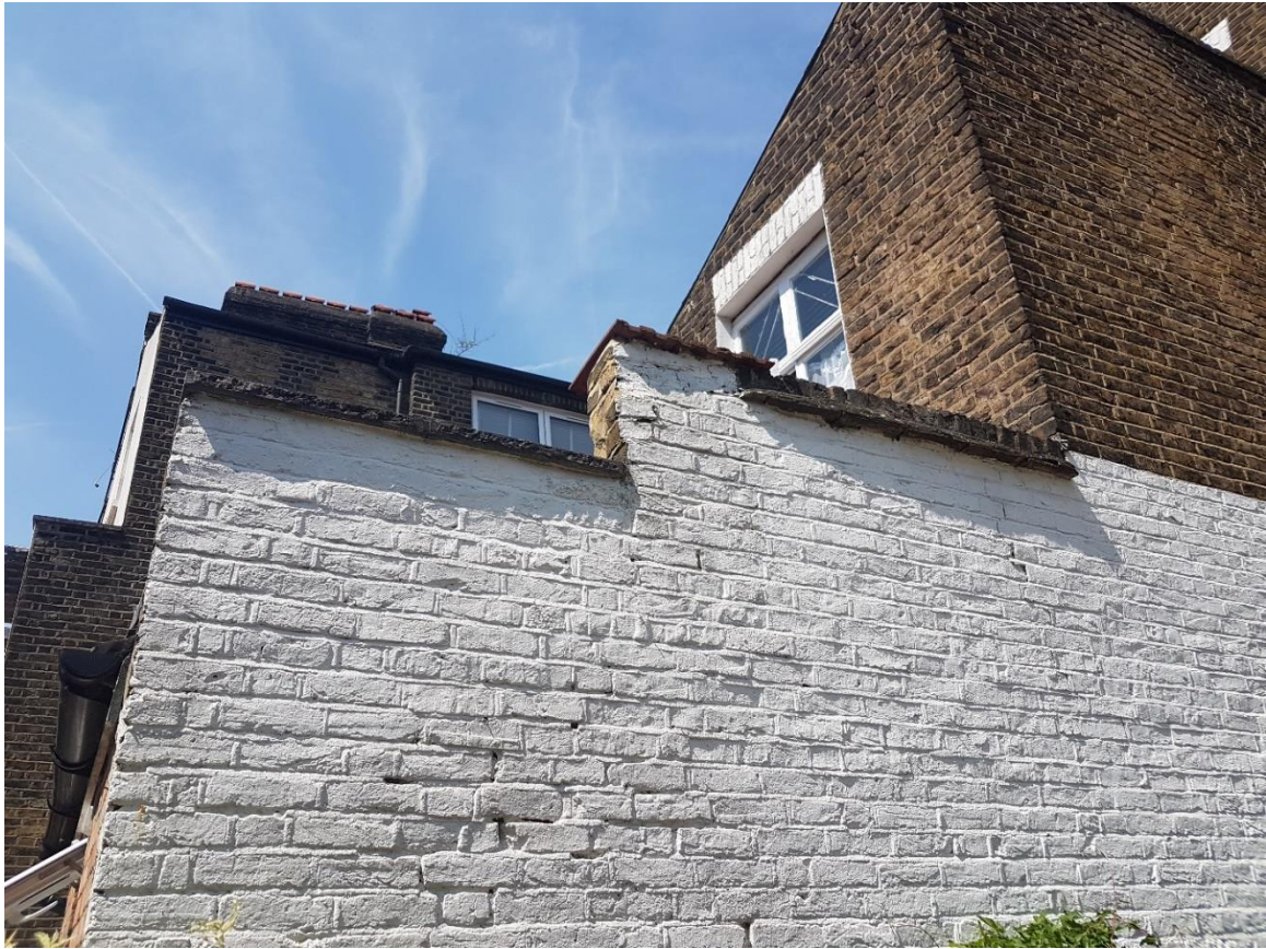
Fig.3 – Rear end of the 9 metres part double part single storey neighbouring rear extension
