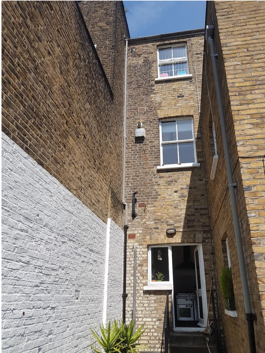
Fig.1 - Rear of 38A Iverson Road - Left hand side massive double storey extension
