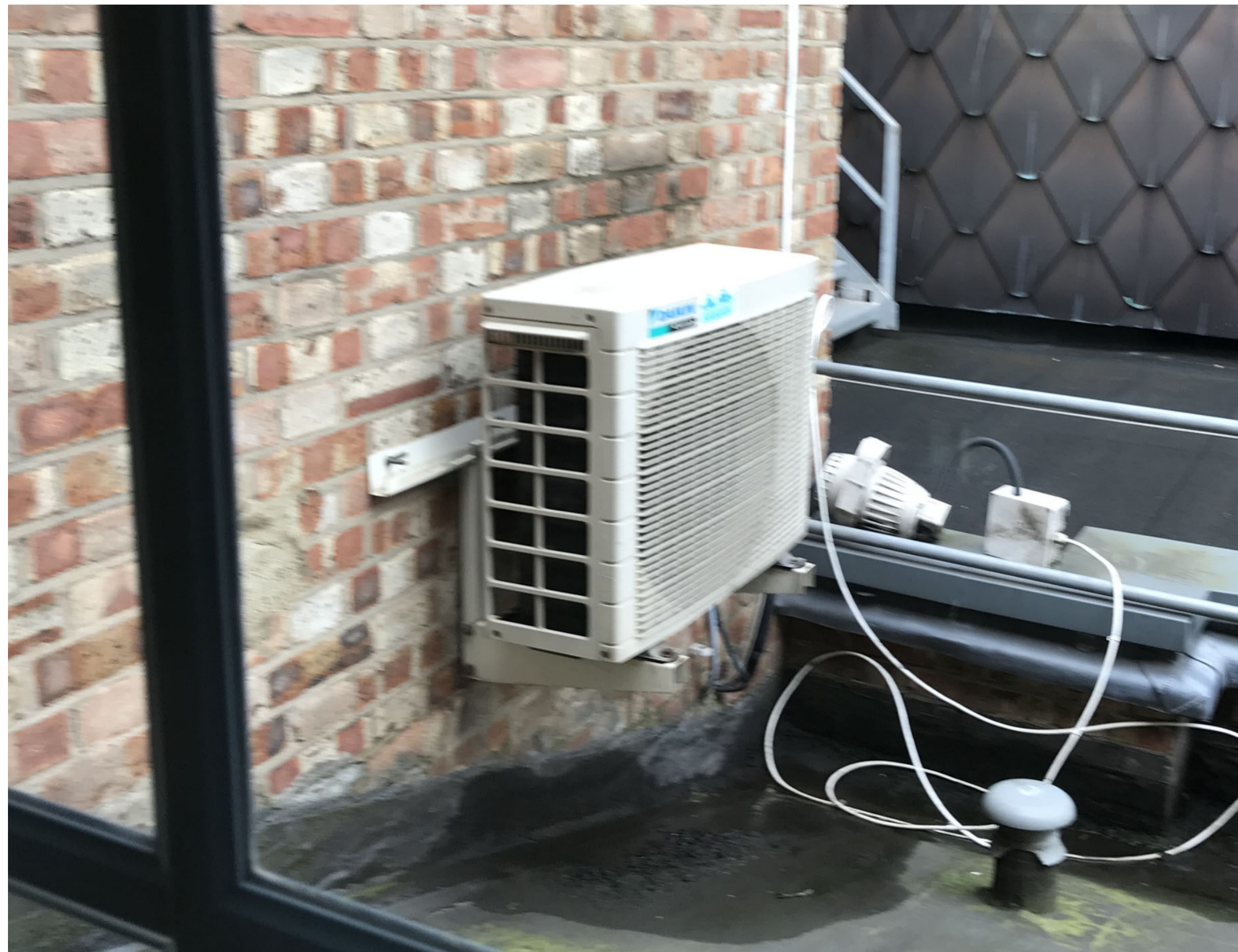
View of Existing Outdoor Units E6 (Air Source Heat Pump) at First Floor Roof Level
