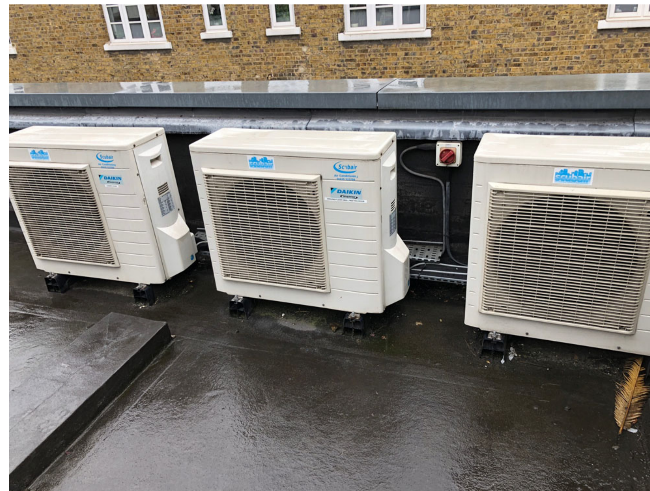
View of Existing Smaller Outdoor Units ASHP E3, E4 & E5
