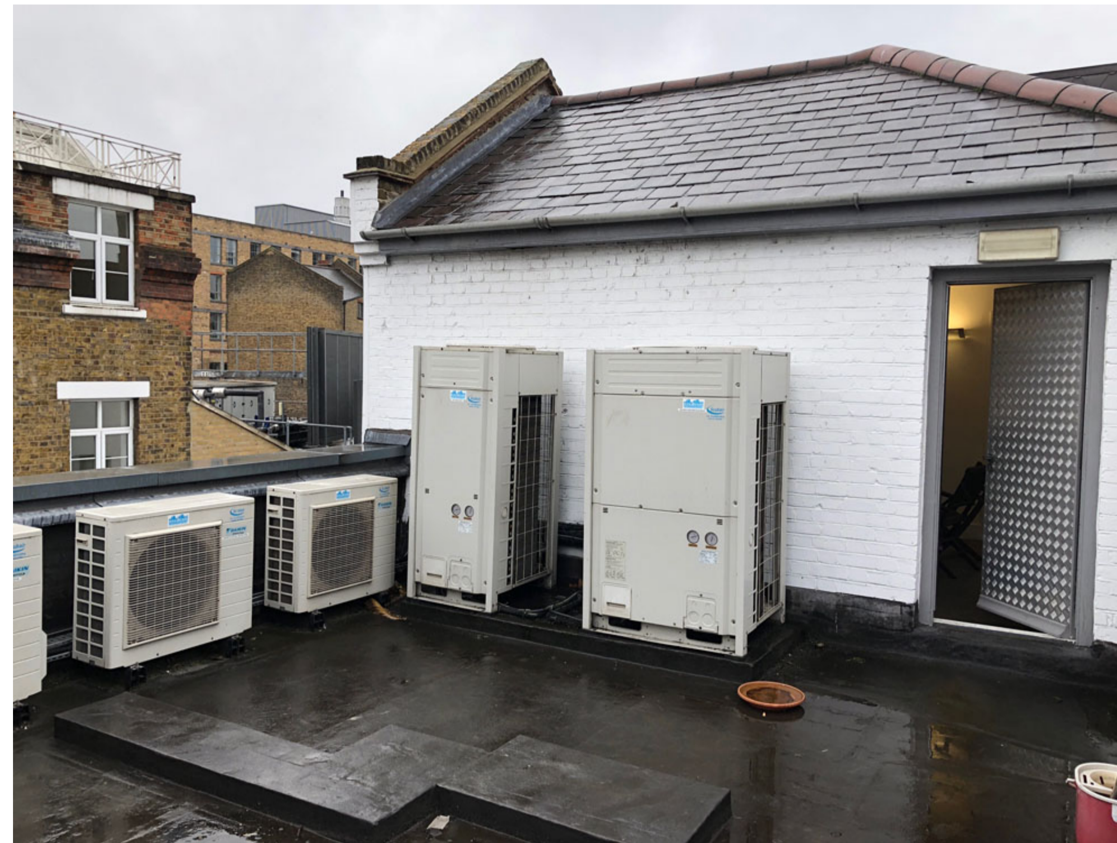
View of Existing Outdoor Units (Air Source Heat Pump) L to R - E5, E4, E3, E2 & E1
