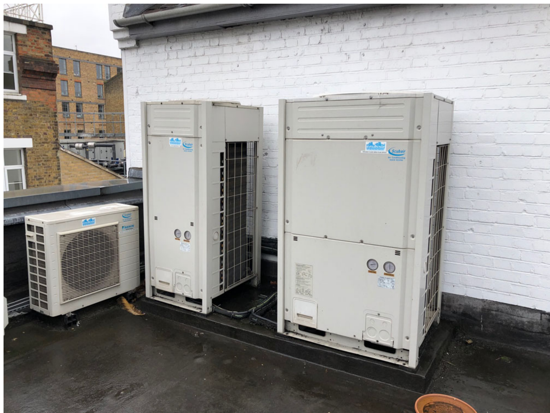
View of Existing Larger Outdoor Units ASHP E1 & E2
