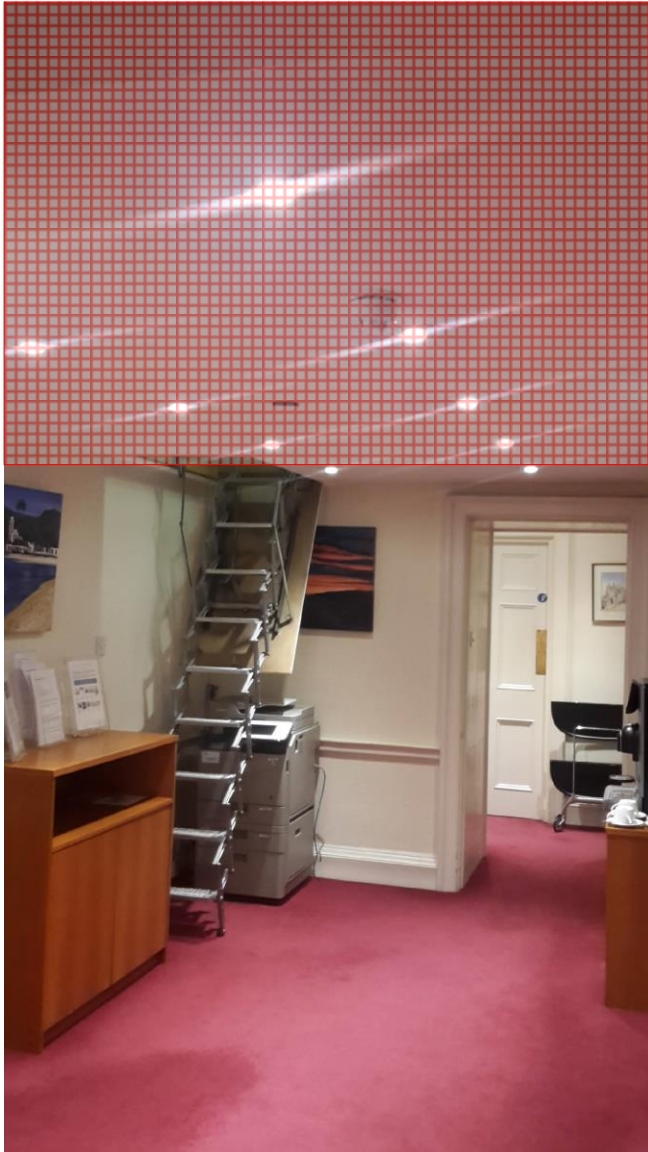
Plasterboard ceiling housing loft storage to be removed to expose vaulted ceiling.
