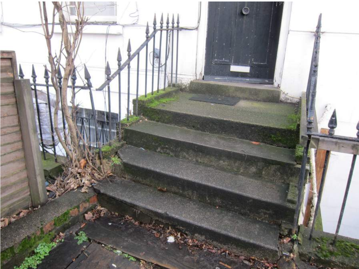
Front steps to 33 Crowndale Road, with sloping steps and missing balusters and finials
