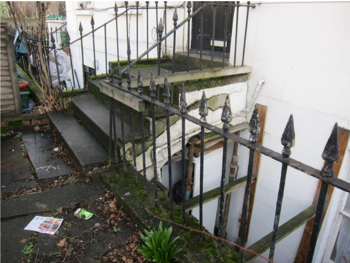
Front steps to 33 Crowndale Road, with propping under collapsed arch
