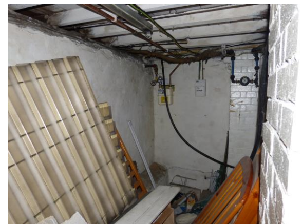
Pic 11 - basement view of incoming services
