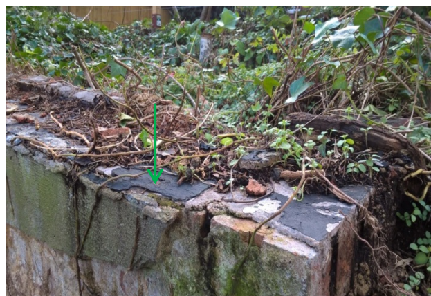
Photograph 4: External – Bitumen to top of parapet walls sampled and found to be negative for asbestos.
