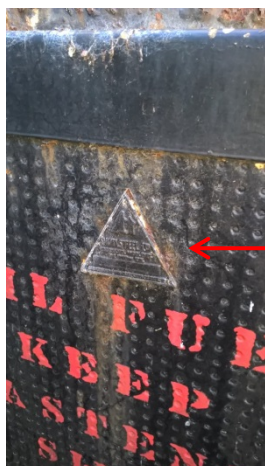
Photograph 3: External – Durasteel panel to external of entrance door to G.01 Oil Store.
