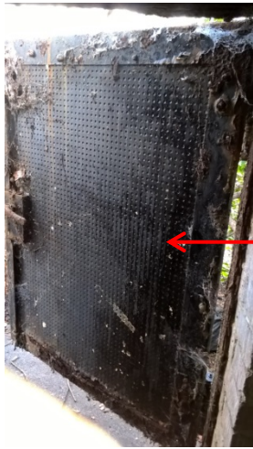
Photograph 1: Ground Floor – G.01 Oil Store – Durasteel panel to internal of entrance door.
