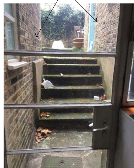
View from the interior to rear garden showing access to garden dominated by un-original extension brick walls.
