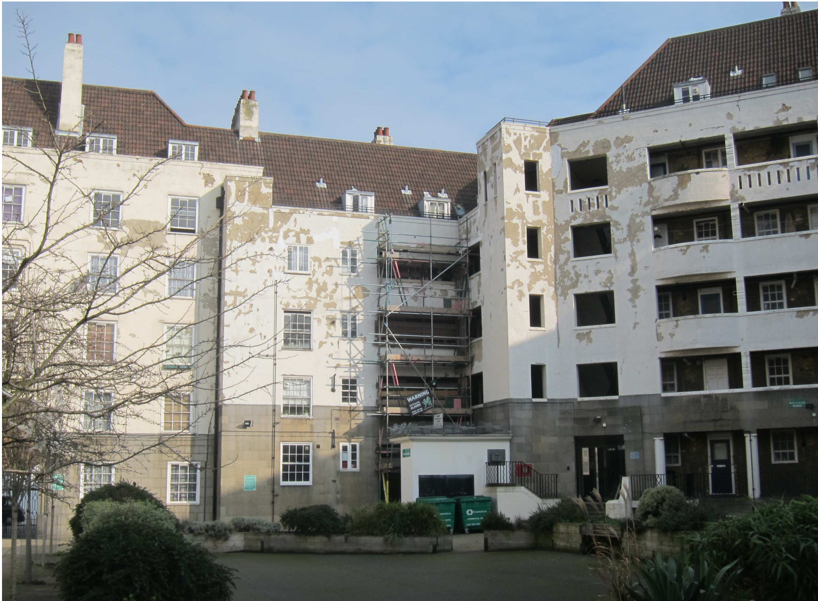
View from courtyard, with scaffolding to protect against falling debris from top floor balcony edge beam
