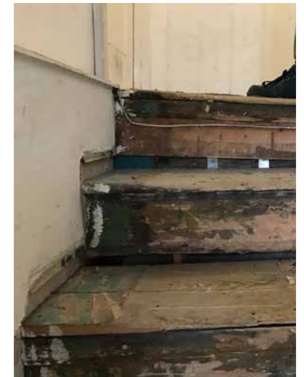
Significant deflection exposes underlying structure
