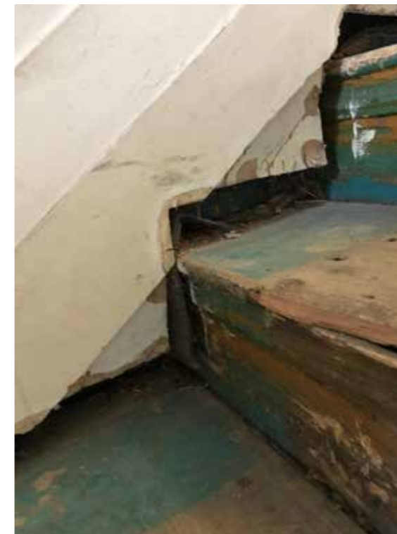
Stair deflection raises significant safety concerns
