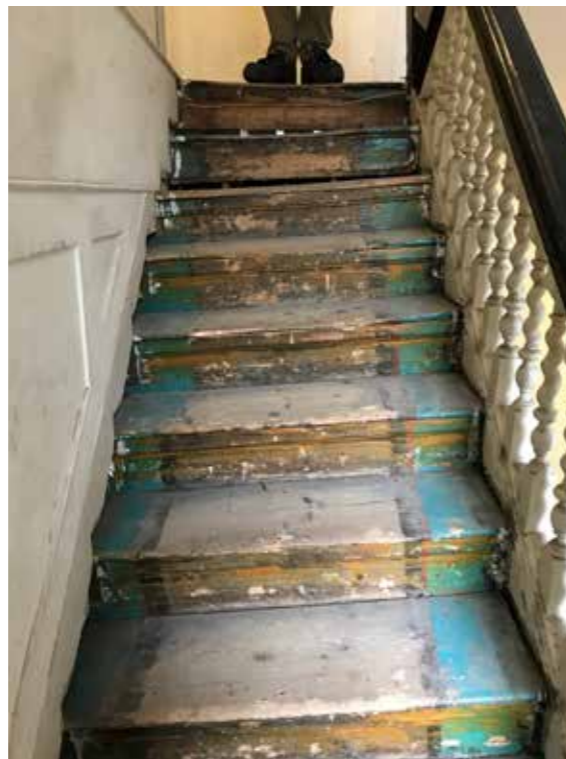
Evidence of severe deflection within the stair wells
