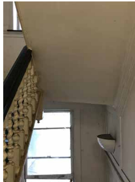
Later plasterboard soffit requires further inspection
