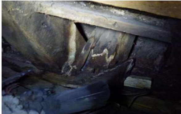
Figure 4.8.11 Rot inside No.26 Roof Space
