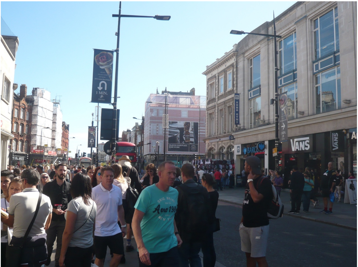
187 Camden High Street during sponsored restoration. Full working scaffold shrouded in 1:1 visual representation of host building, with 10% inset sponsorship area, in the Camden Town Conservation Area.
