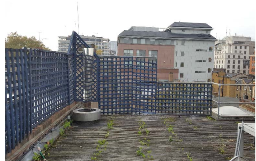
Existing condition of the roof terrace, looking West towards Red Lion Square
