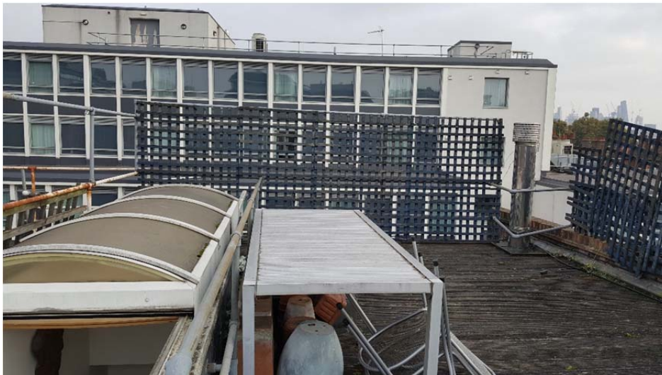
Existing condition of the roof terrace, looking East towards Premier Inn building
