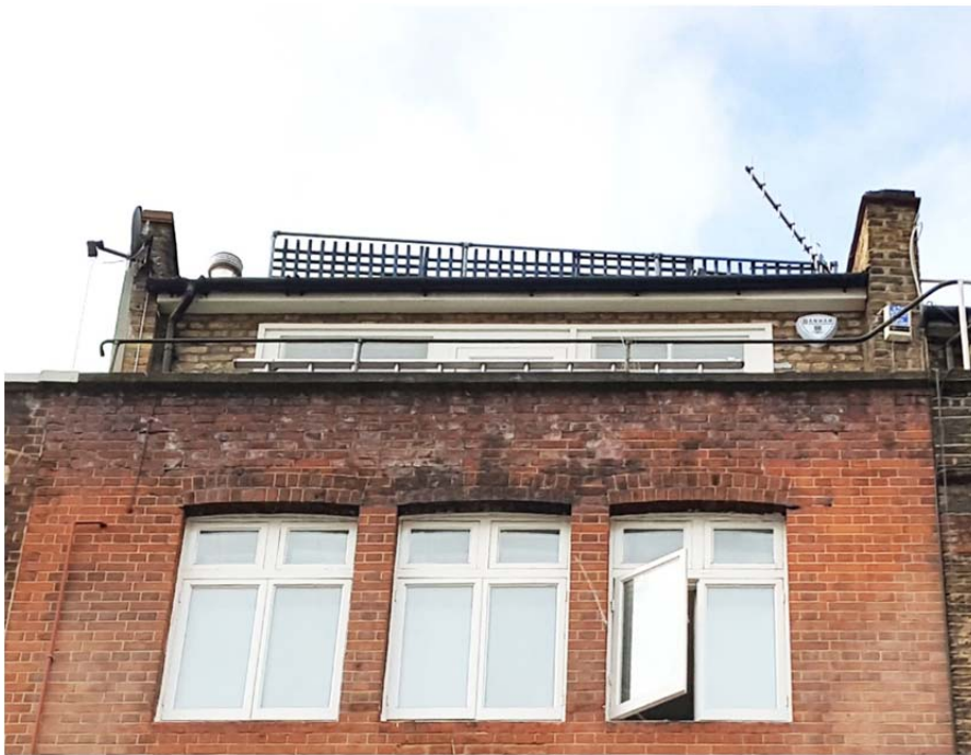
Existing front elevation with timber lattice screen on the roof terrace, fourth floor metal balustrade and deteriorating stone coping. Water damage visible on the top of the brick wall.
