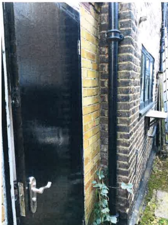
Figure 7 The west wall of the existing rear extension is set in from the side of the outrigger. It is proposed to move the extension wall outwards to make it continuous with the outrigger wall.
