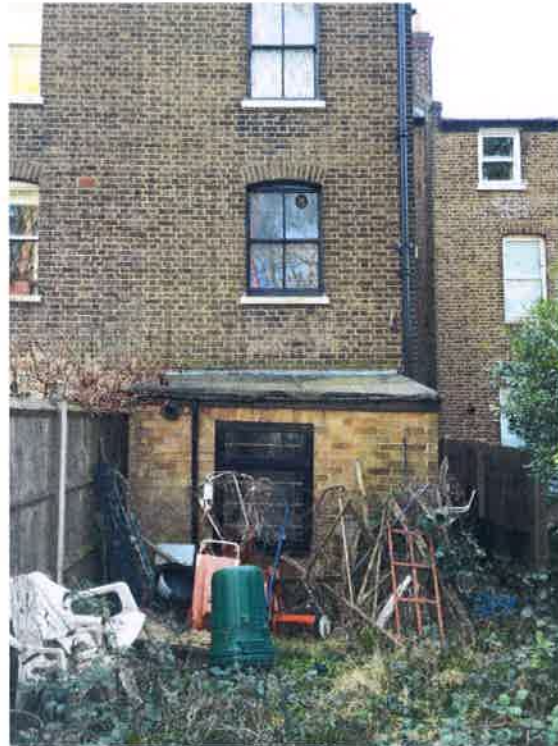
Figure 3 The rear elevation as existing; the rear extension provides a poor connection to the external amenity space.
