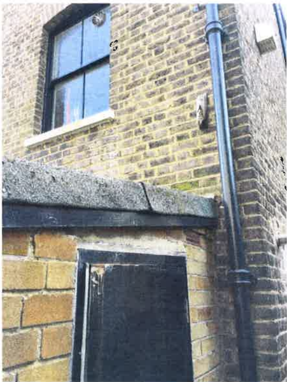
Figure 5 The existing roof to the rear extension is of a poor quality and detracts from the rear elevation of the original house.
