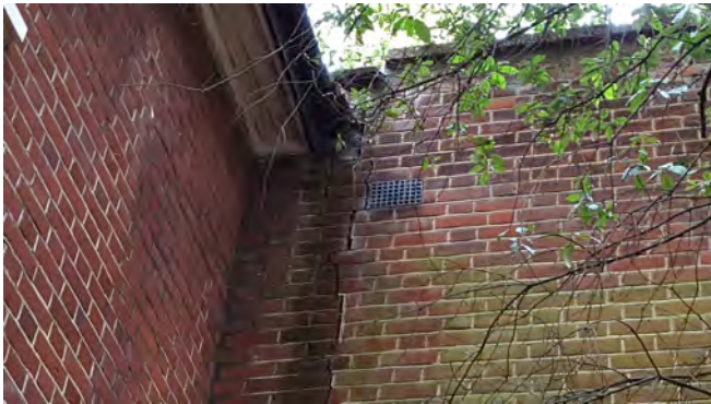
Crack in garage wall
