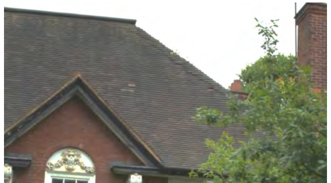
Front facing roof with broken tile
