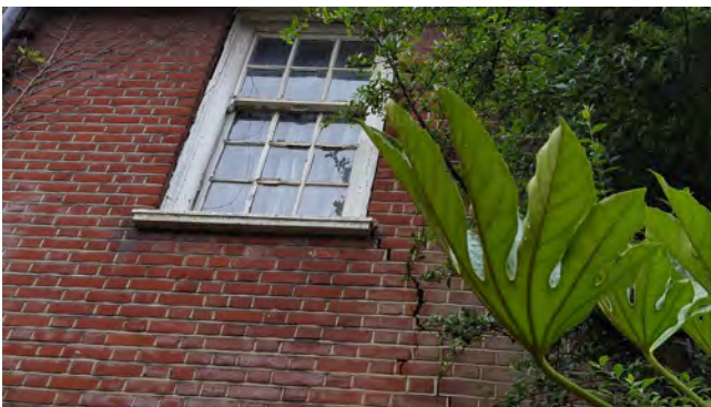
Crack in the wall on the front façade
