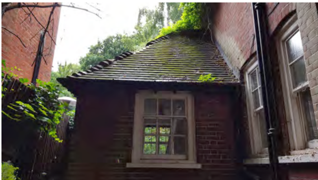
Extension with missing tiles on roof ridge
