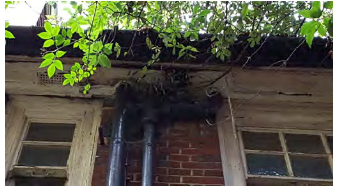
Gap in soffit covered by tree branches
