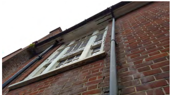
Hole in the south-west facing soffit
