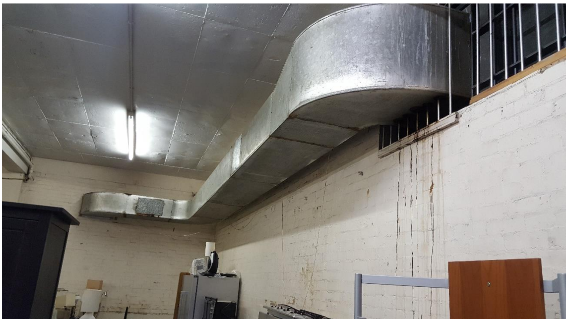
Image 10 – ductwork routed through the building
