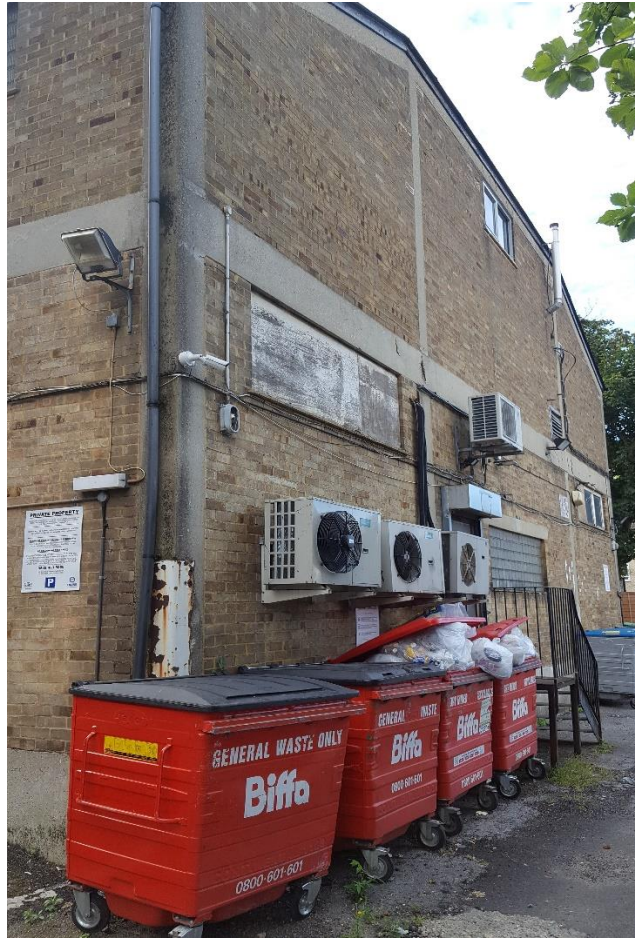
Image 5 – Air condensers and bin storage along rear elevation
