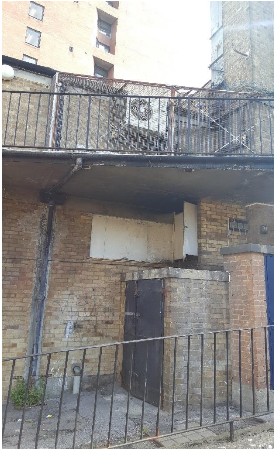
Image 3 – Air condensers present at upper ground floor level
