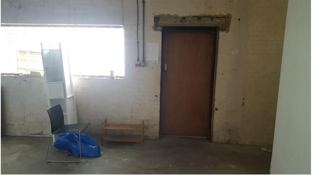
Image 13 – Unit in need of repair
