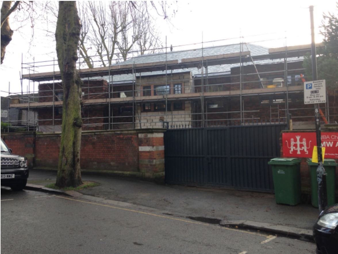
3. View towards partially completed house (hips and pediment still to be constructed)
