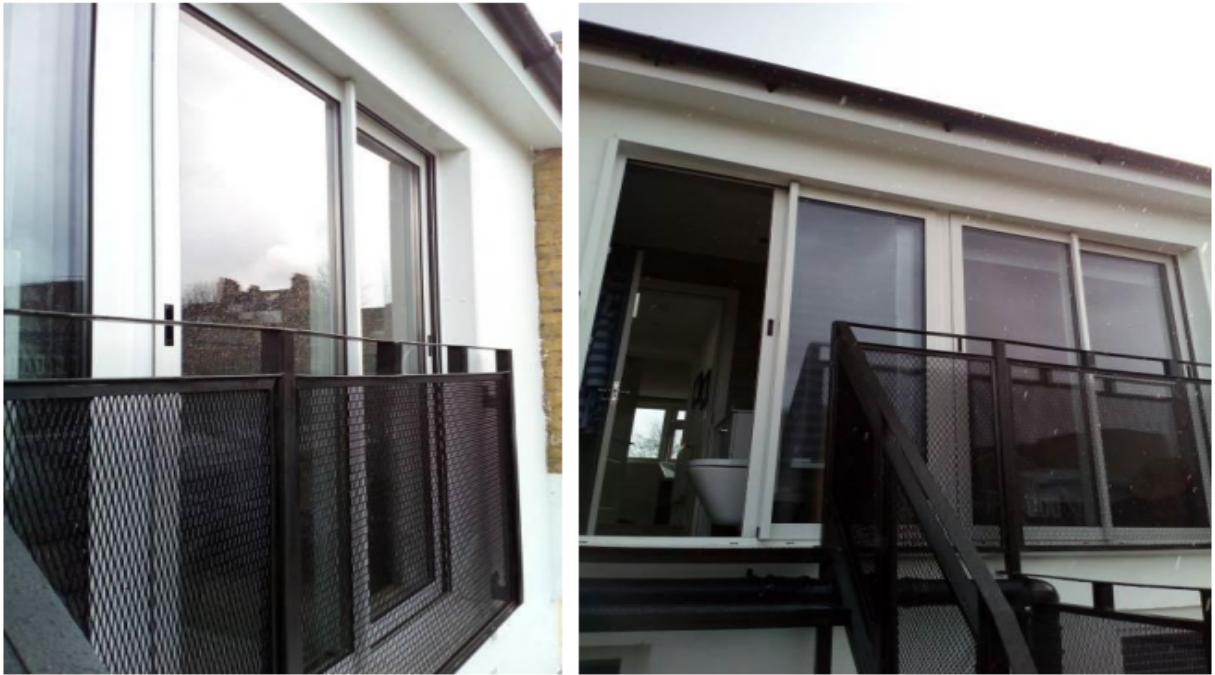
Photograph 1. Existing rear dormer doors/windows and existing mesh Juliet balcony to be removed.
