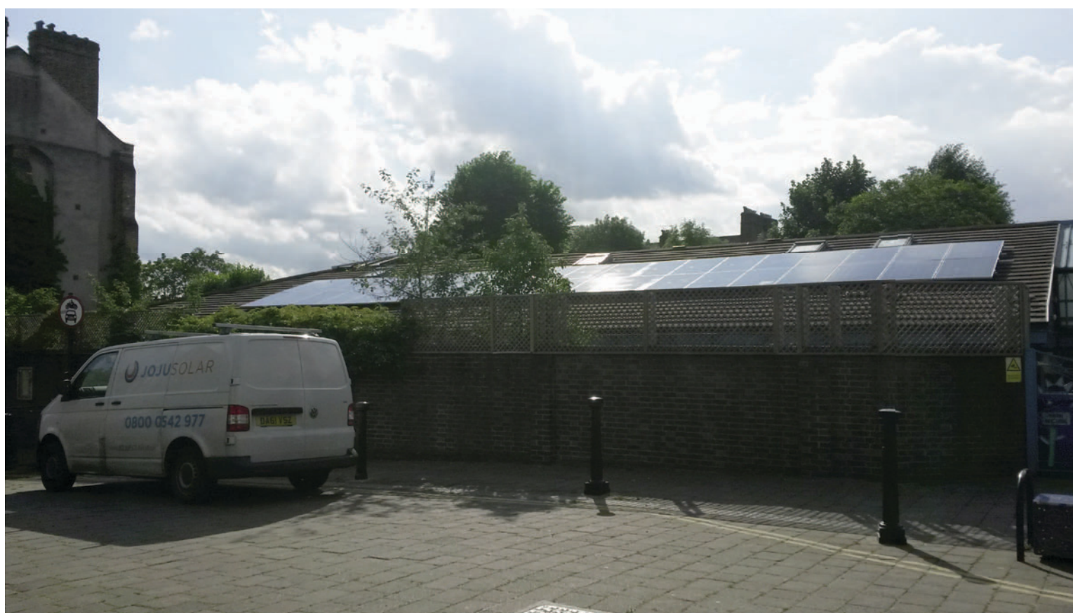
PV solar panels at Eleanor Palmer Primary School, Kentish Town
