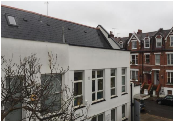
3. Photograph taken from no.1 living area showing roof of no.3 and no.2 (including existing roof light at no.2)
