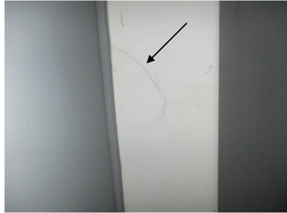
Cracking in kitchen
