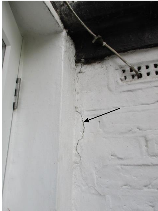
Cracking at rear addition junction
