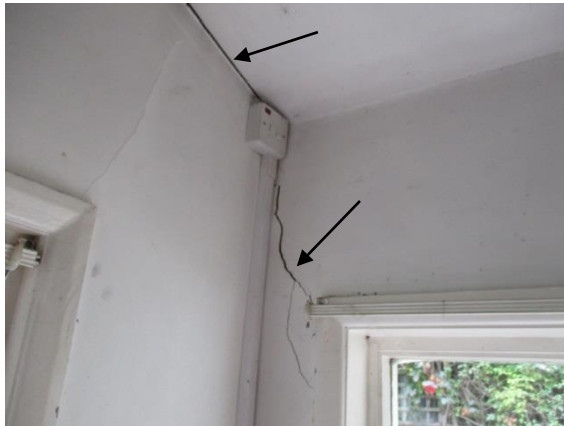
Cracking in utility room
