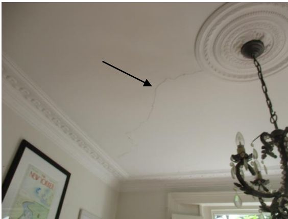
Cracking to ceiling in lounge
