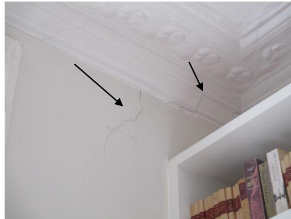
Cracking in lounge
