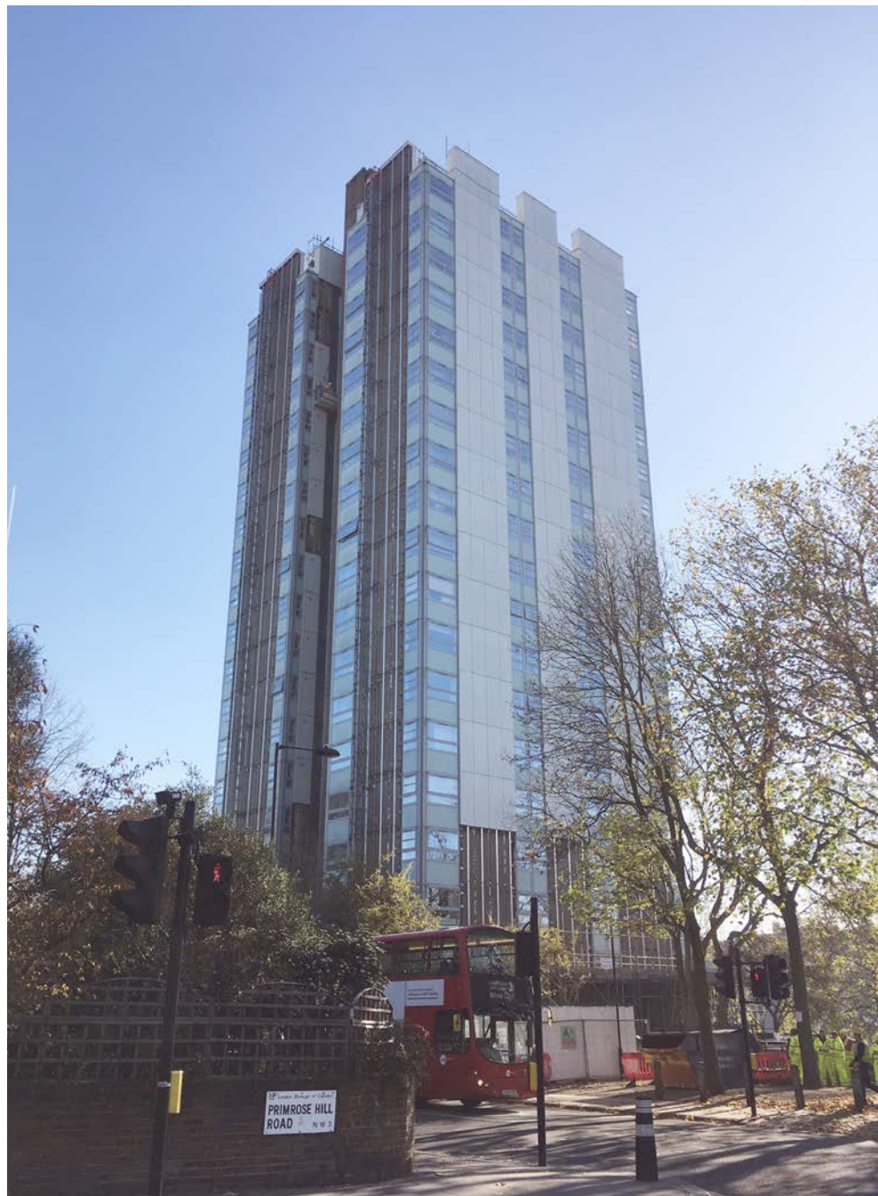
V9 - Existing Blashford Tower, mid cladding removal (junction of Primrose Hill Rd & Adelaide Rd)
