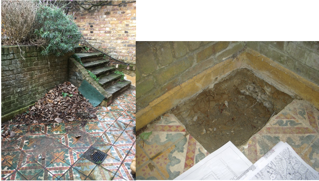
Photo 2 (left): Showing the steps leading up from the patio to the level T1 is growing on, and shows the patio retaining wall.
