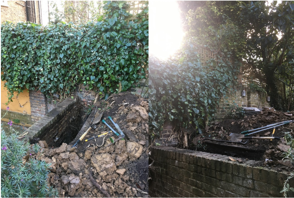
Photo 4 (left) and Photo 5 (right): showing the size and positioning of Trial hole 2 (its position is shown on Figure 1 – Tree Constraints Plan - in section 9 of this report).
