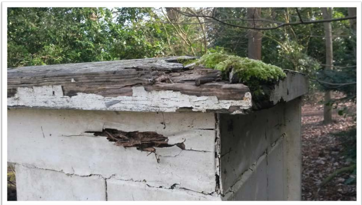
Fig. 3 North Abutment showing progressive decay.
