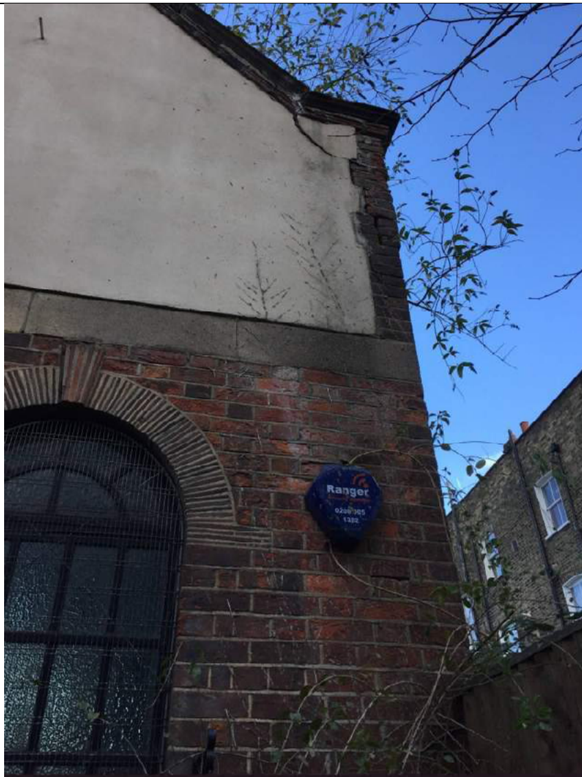
Plate 3: Crack along facias and brick.
