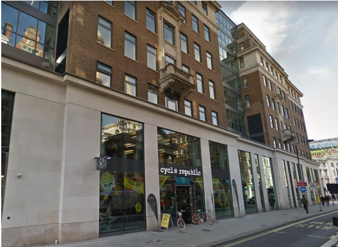
Photo of the North Elevation showing the Louvres located on the ground floor and the first floor (Bloomsbury Way)
