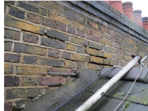
repointed brickwork harmful
