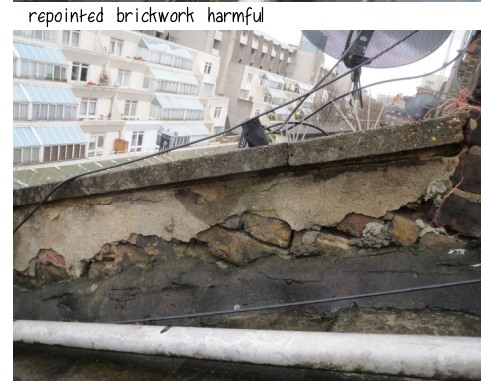
party wall - poor
