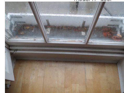
bottom rails require maintenance
