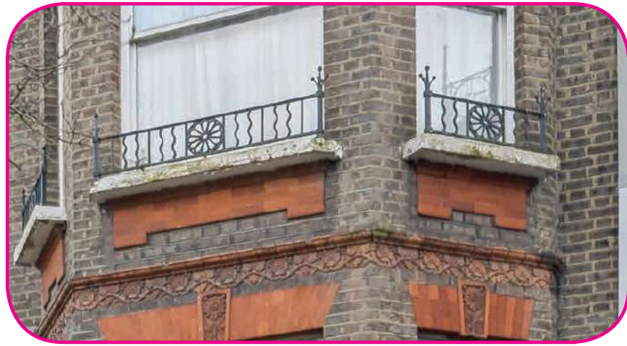
DETAIL 1 REFERENCE IMAGE - PICTURE OF EXISTING LOW LEVEL RAILING TO WINDOW APRONS
