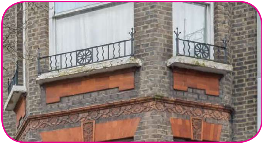
DETAIL 1 REFERENCE IMAGE - PICTURE OF EXISTING LOW LEVEL RAILING TO WINDOW APRONS
