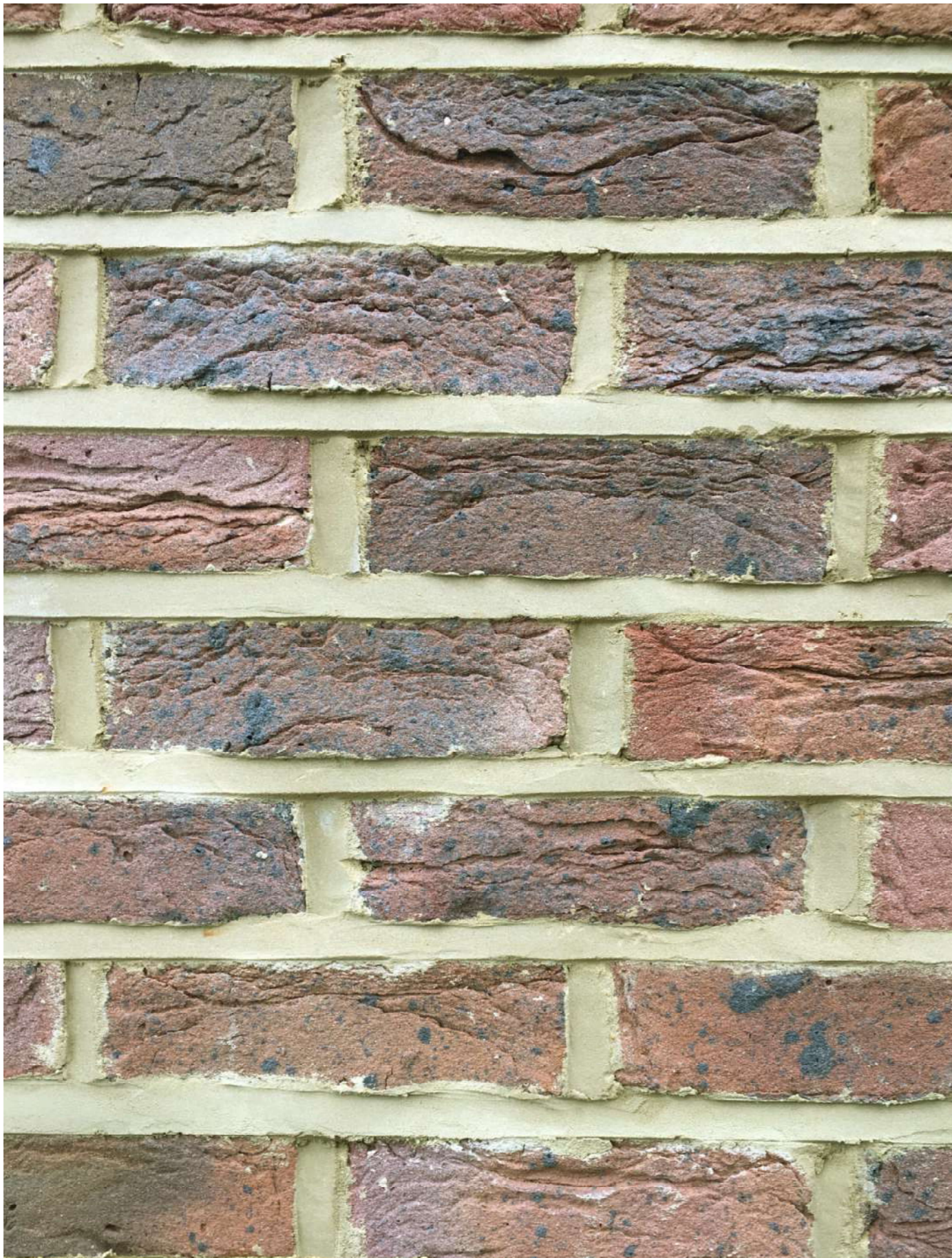
PROPOSED NEW BRICK 65MM METRIC BRICK FITZJOHNS NOBLE PICTURE OF SAMPLE PANEL FOR APPROVAL
