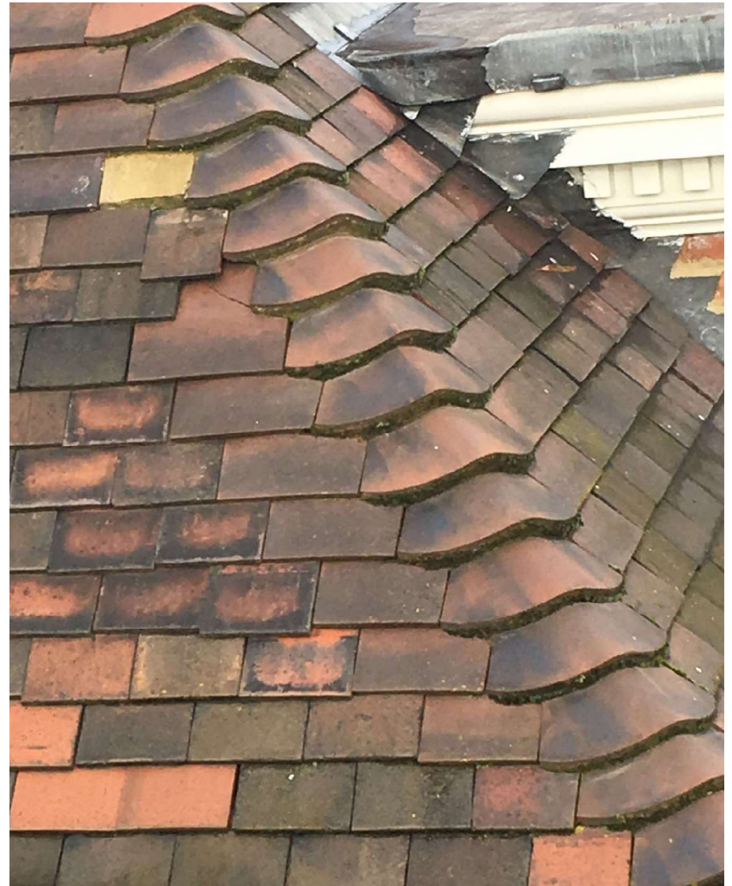
EXISTING CLAY TILES TO THE ROOF OF NUMBER 13 FITZJOHNS AVENUE NOTE: PICTURE SHOWN FOR REFERENCE ONLY. PICTURE SHOWS FULLY WEATHERED CLAY TILES
