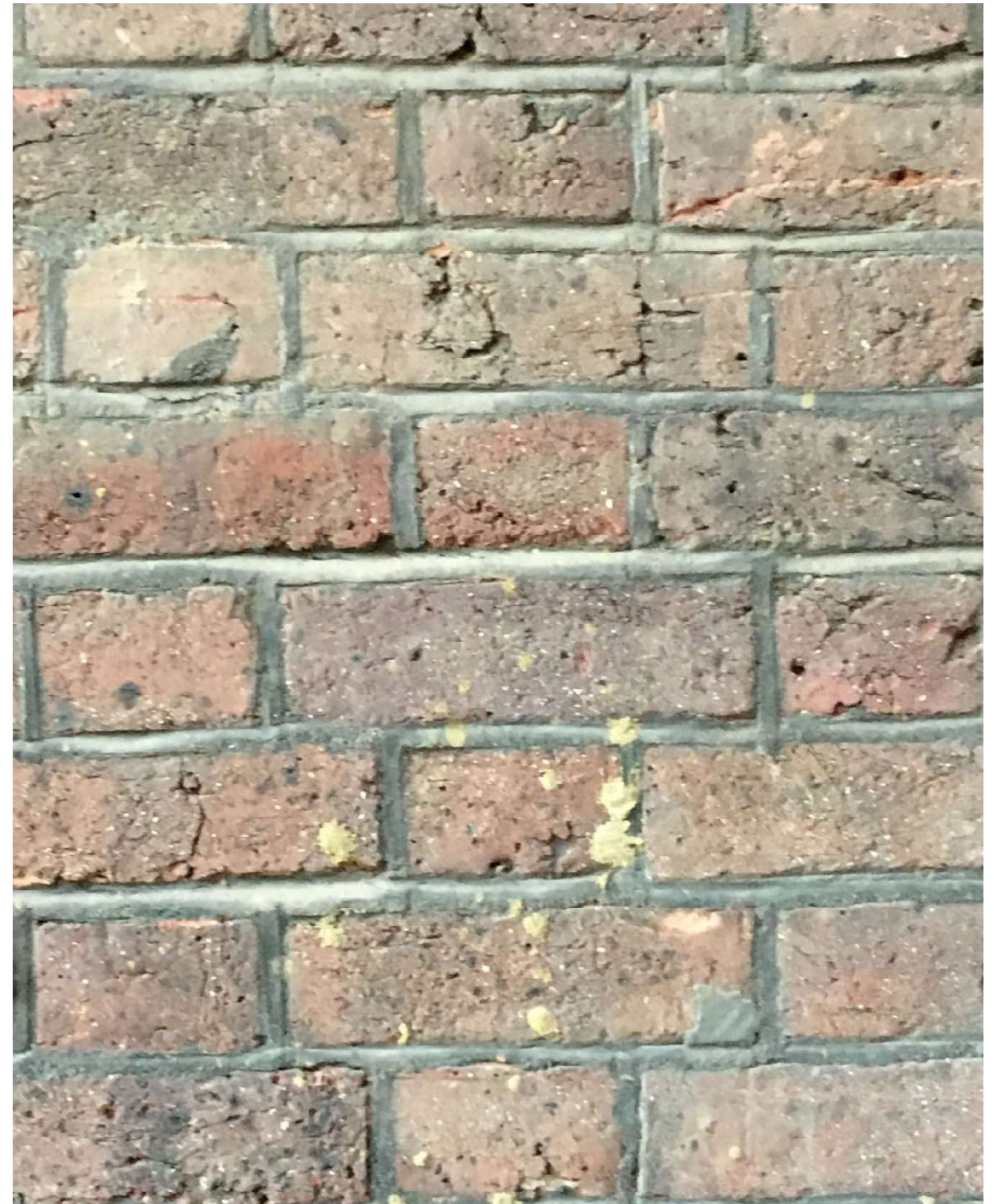
EXISTING BRICK TO BE CLEANED AND RETAINED NOTE: PICTURE SHOWS UNCLEANNED BRICKWORK AND MORTAR JOINTS
