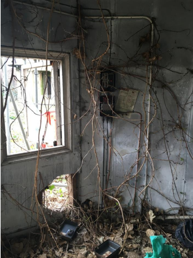
Fig 19. Asbestos and services
