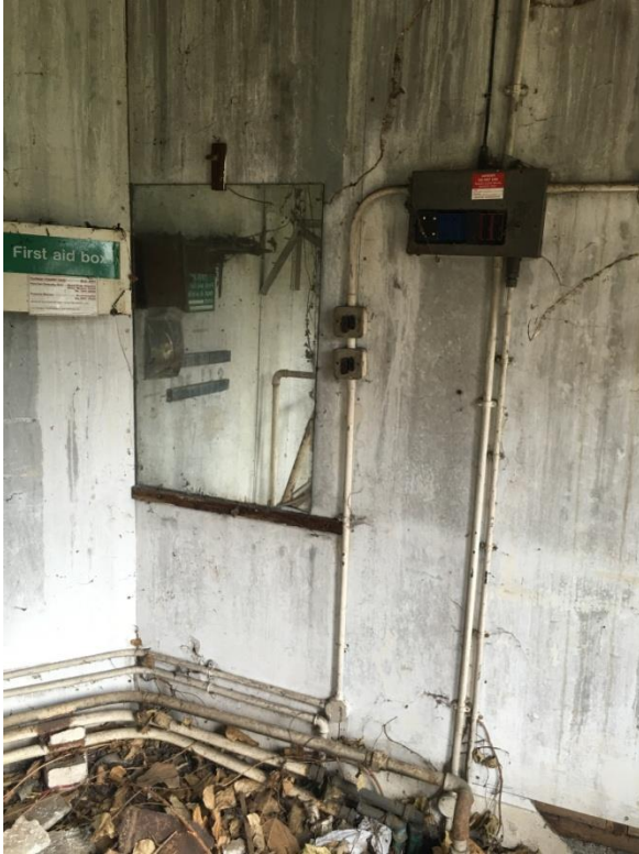
Fig 17. Asbestos lining and services
