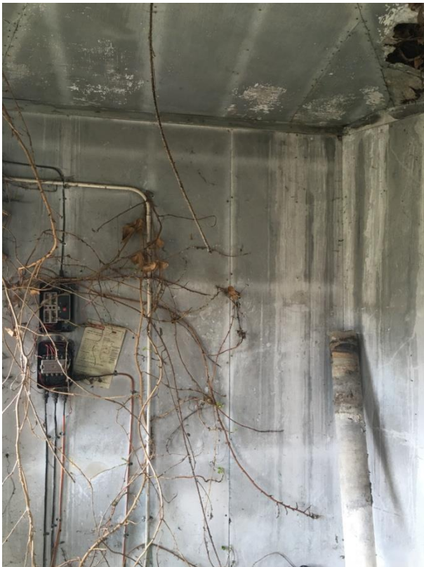
Fig 18. Asbestos and services
