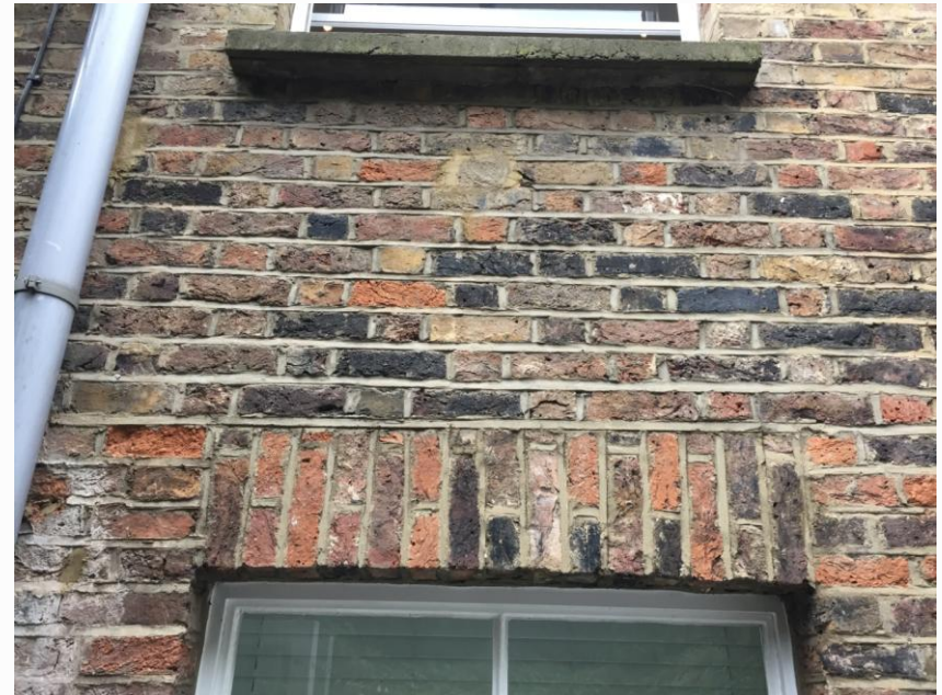
Fig 33 The panel of brickwork between the rebuilt window head at basement level and the concrete cill of the 1 st floor window.
