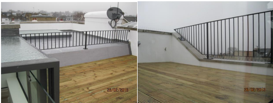
Existing Roof/Terrace Photo - 1x Retractable rooflight and 1 x rooflight - 1.1m Safety railing at the rear elevation
