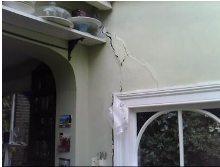
FIGURE 05 Summer Room - cracking above window.
