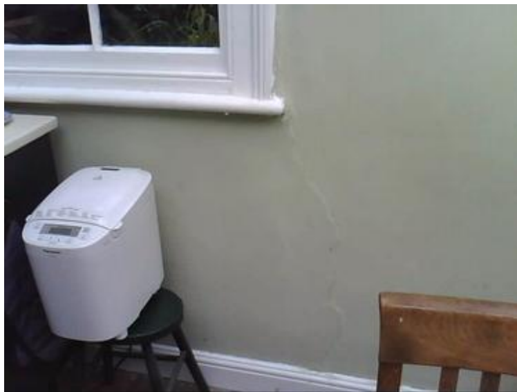
FIGURE 06 Summer Room - cracking below window
