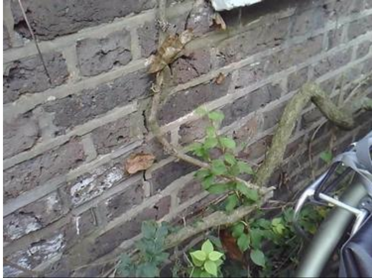
FIGURE 04 Left Hand Elevation - cracking below window.
